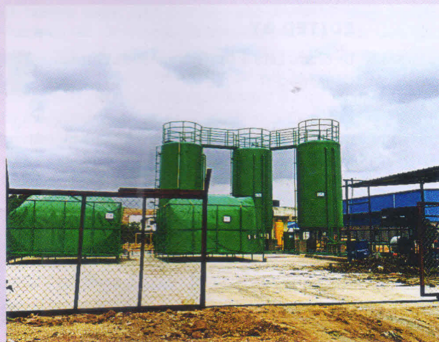
5 ton/day biogas plant at the Jawahar Nagar MSW Dump yard in Hyderabad
