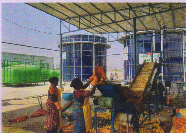
10 ton/day biogas plant based on AGR technology at the Bowenpally Vegetable Market Yard
