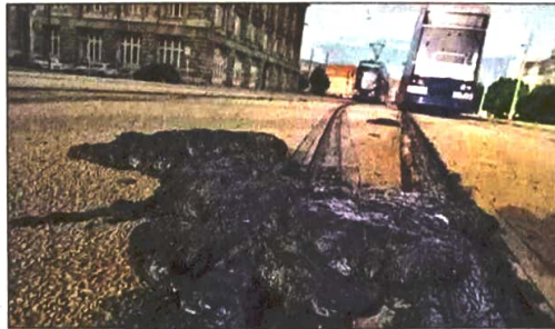
The heatwave caused significant damage to the tram infrastructure in Leipzig, Germany, on Saturday. (AP)
